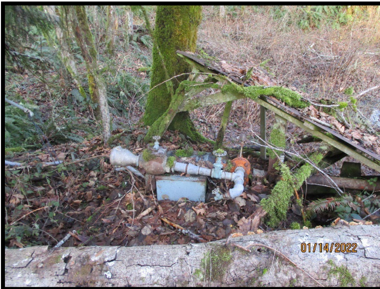
Photograph 6: Remains of old pump system adjacent to the manmade pond located along the southwest property boundary.
